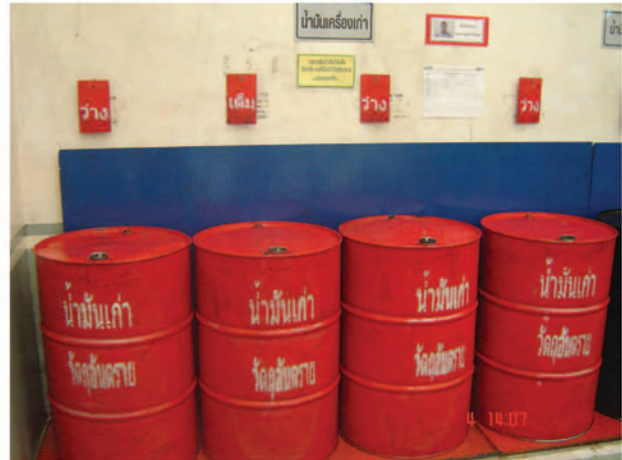
Proper Fuel Storage
